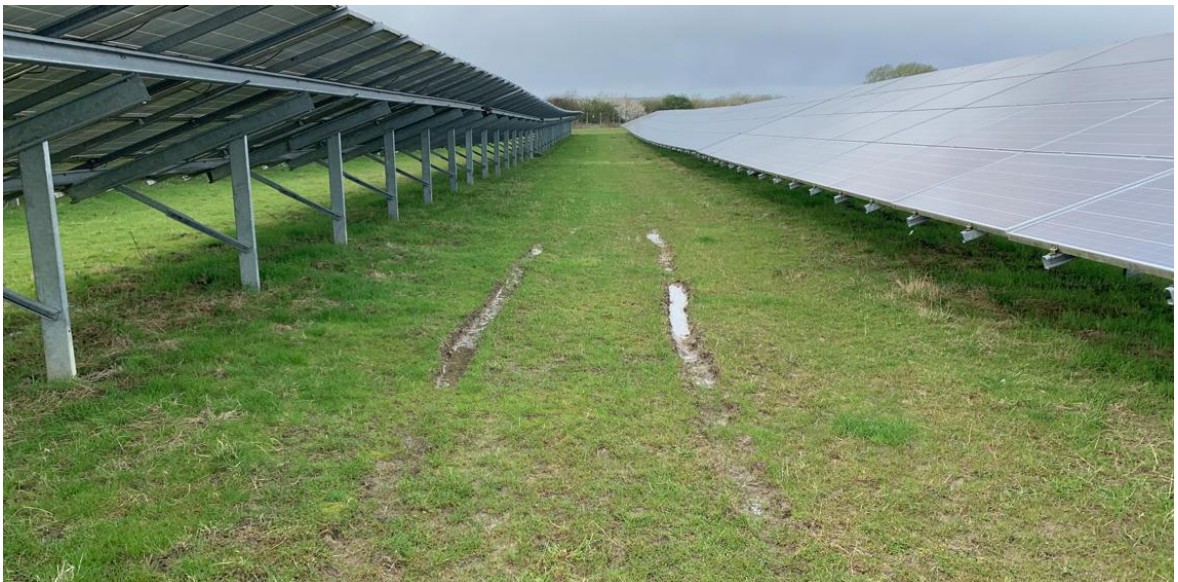
Plate 11-41 Example of Minor Ruts Caused by Vehicles
